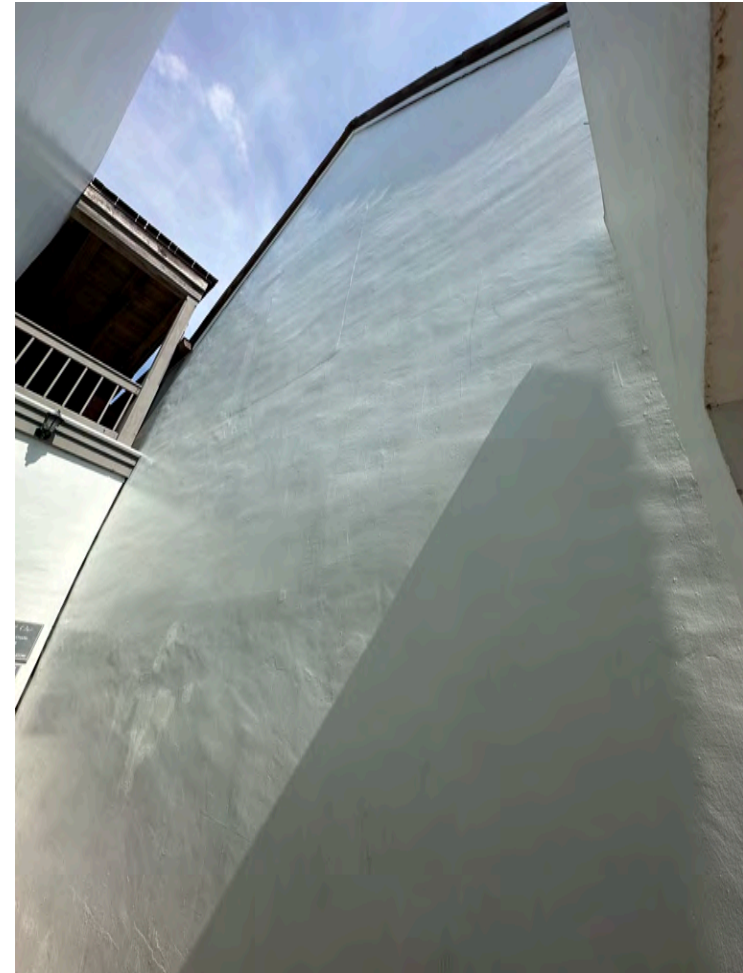
D: West Wing, N facade, looking SE and up
